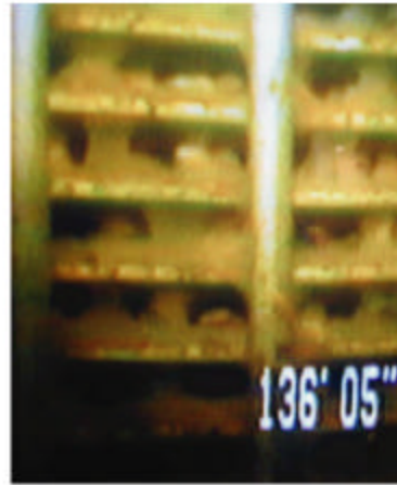
Fouled Well Screen
